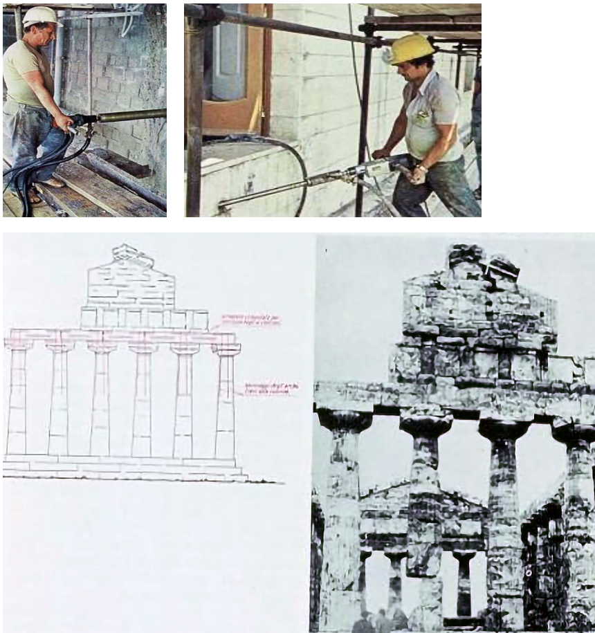
Fig. 68. Reinforced. Problems in Paestum. From F. Lizzi, The static restoration of monuments , Sagep Publisher, Genova 1982.
