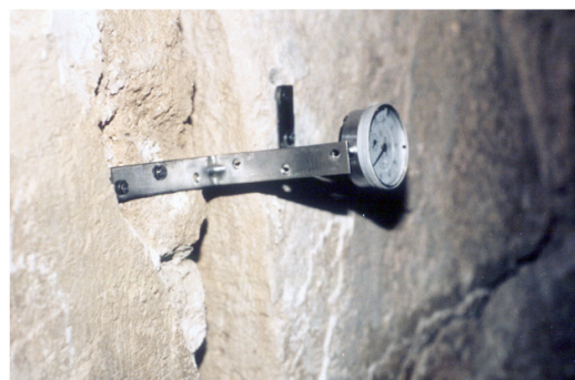
Fig. 43. San Bartolomé Parish Church. Structural consolidation. Foundation reinforcement through micropiles. Sewed of factories. Follow-up through instrumentation. Susana Mora. Tarazona de la Mancha, Albacete 2000.
