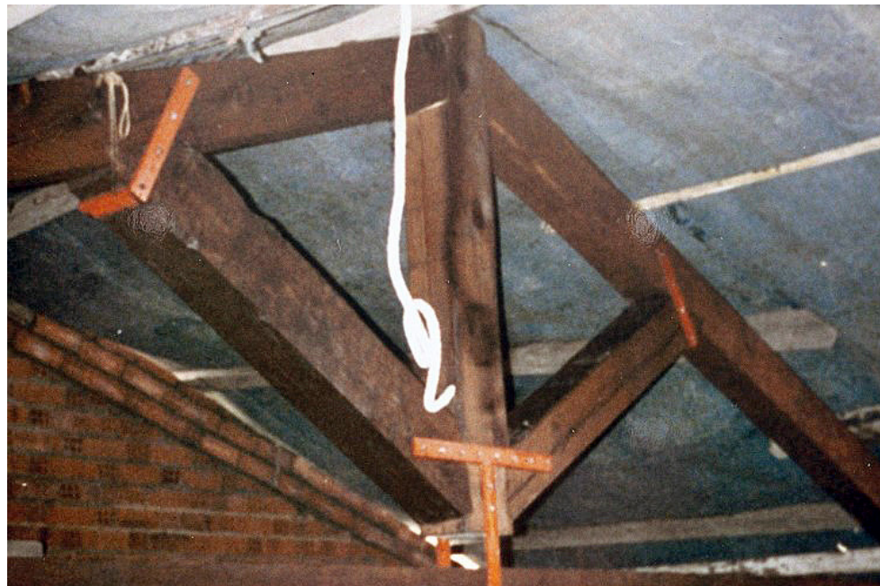
Fig. 26. Capitulo roof structure of Gradefes Monastery. Restoration and photo by Susana Mora, 1989.
