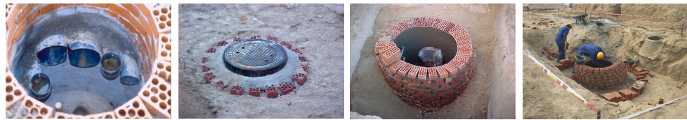
Fig. 55. Circular drainage well. Photos by Celia Barahona.
